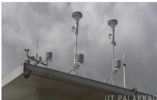
Air quality measurement station
