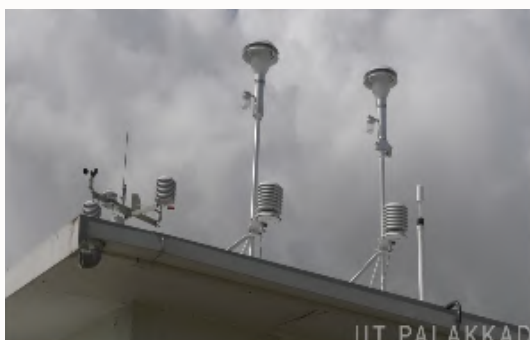
Air quality measurement station
